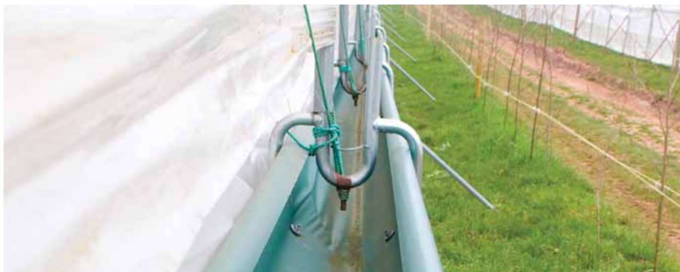
Good guttering is vital to capture rainwater
