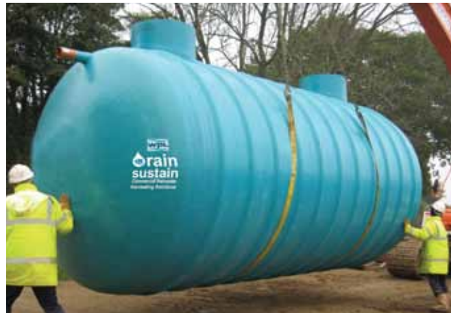
Figure 5 → Examples of underground storage tanks
