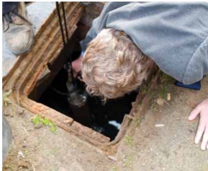
In underground storage tanks ensure you can access the pump for maintenance
