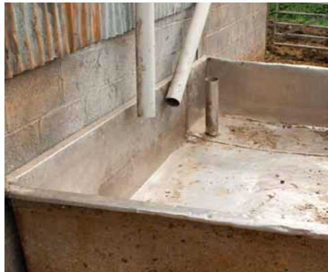
Roofwater enters the drinking trough and a level overflow takes it to the surface water drains
