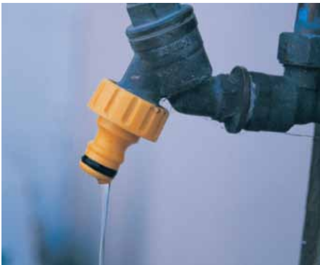
Before considering new sources of water supply identify where you may have leaks first
