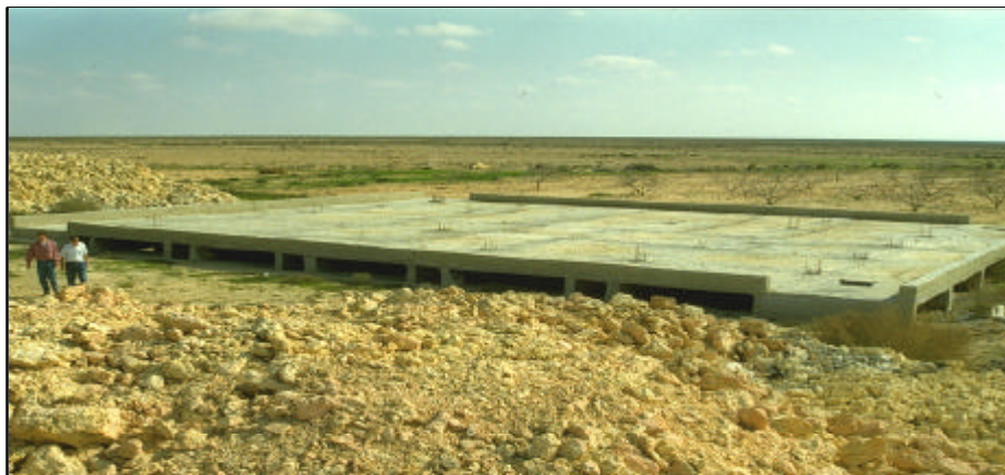
Figure 7: Concrete cistern of 3000 m 3 storage volume, constructed in Marsa Matruh area, NW Egypt . Photo: Prinz
